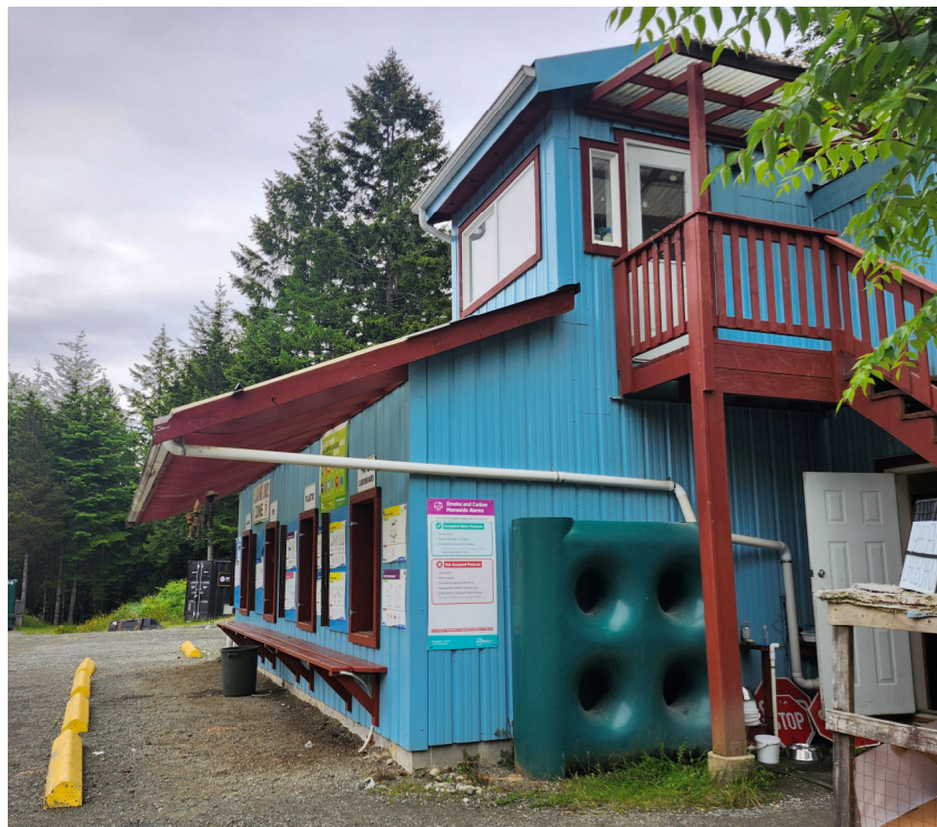
Figure 3. Rainwater collection systems such as this one at the Cortes Island Recycling Centre can supplement or provide water supplies on properties without a well or nearby surface water source.
